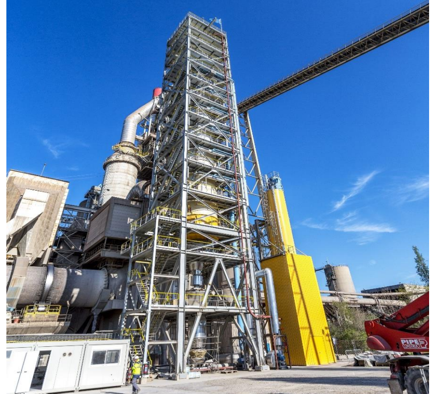
LEILAC project: Lixhe, Belgium
